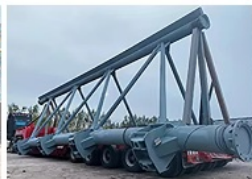
9. Spray paint and galvanize steel structure according to technical requirements of drawings
